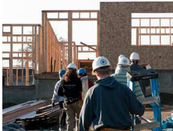
11 The Rainier Vista phase 1 project features retrofit of existing rental housing into a mixed-income community of rental units, condos, and houses—Seattle Habitat
