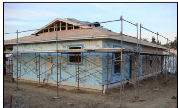
3. ONE INCH EXPANDED POLYSTYRENE FOAM APPLIED TO OSB SHEATHING TO PROVIDE CONTINUOUS THERMAL BREAK AND ADDITIONAL R-5 WALL INSULATION
