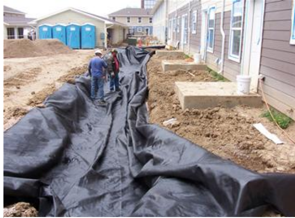
12 Water runoff drains at Bails Townhome Community— Metro Denver Habitat
