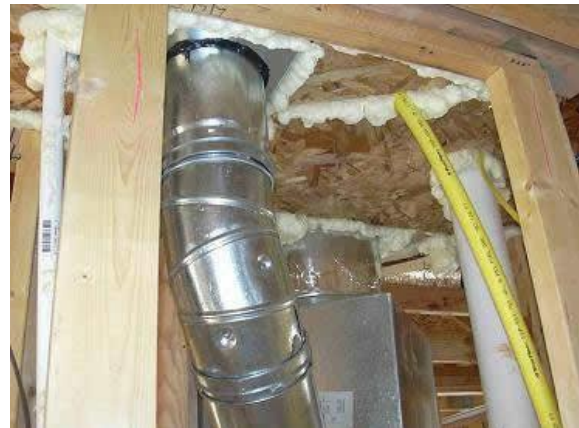
7 Sealed ducts in conditioned space--TriState
